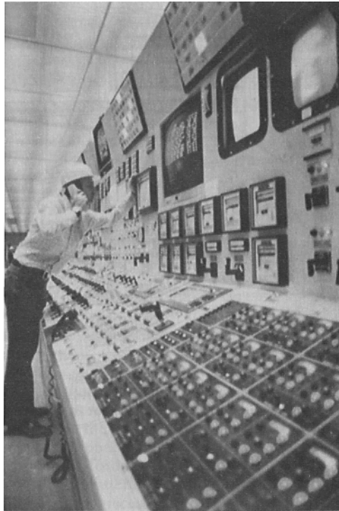
FIGURE 1 Long panelboard containing indicators and controllers used in large processing plant. Generally this type of panel was used in the early 1970s. The very beginnings of the cathode-ray tube (CRT) displays for annunciators are indicated by the CRTs in the upper right-hand portion of the view.
